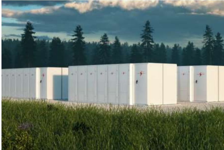
Figure 14 Exemplary representation of the battery storage unit installed. Figure taken from: [29].
